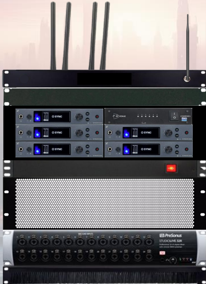
MAIN RACK (FRONT)
