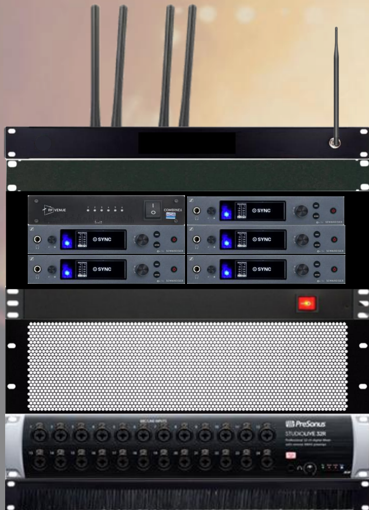
MAIN RACK (FRONT)
